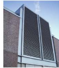
ARCHITECTURALLY LIT LOUVER PANELS
