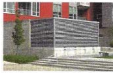
LOUVERED MECHANICAL SCREENS
