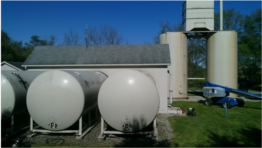
Pressure filters and aerator at the Cherry Tree WTP
